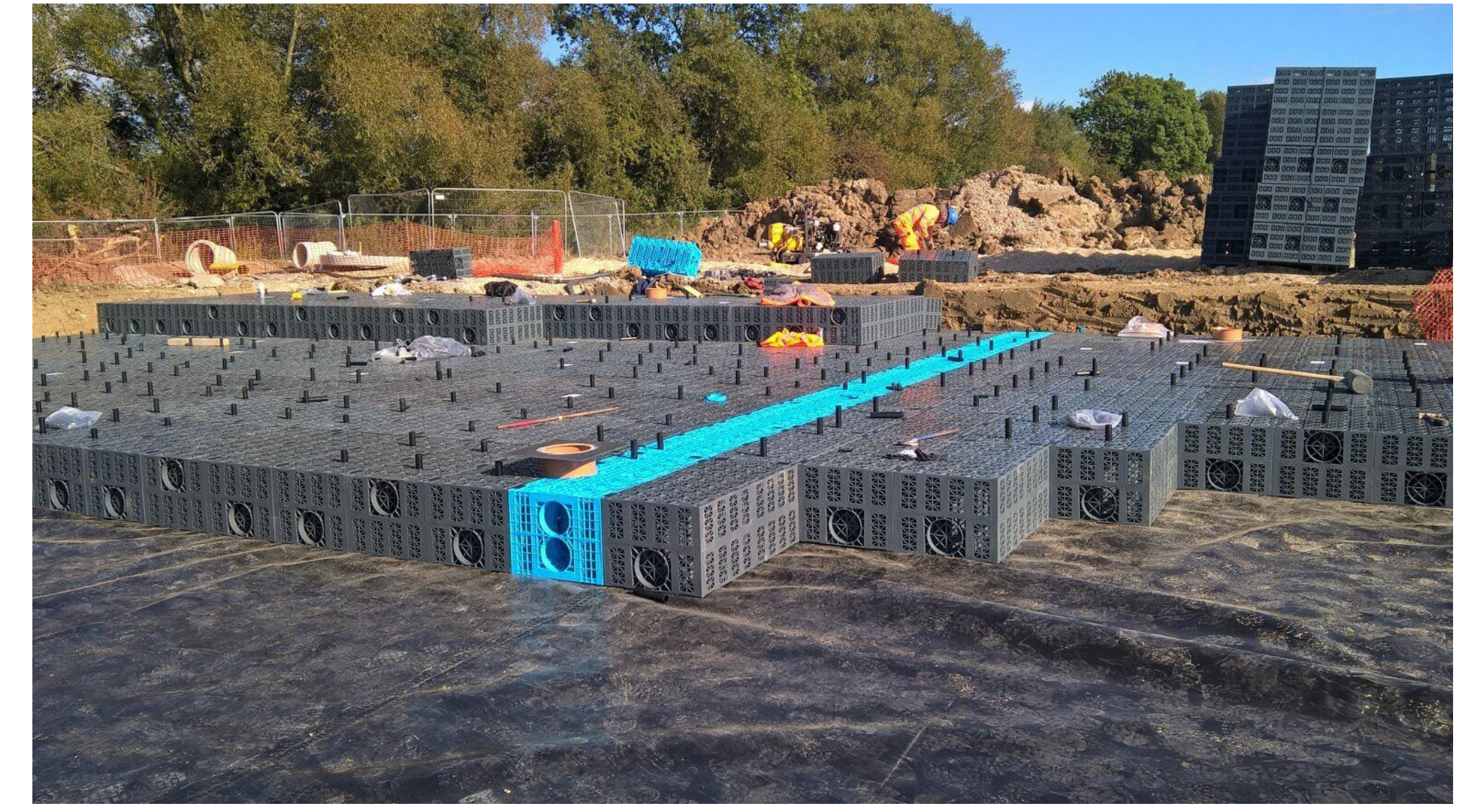
Sustainable Drainage System (SuDS)
